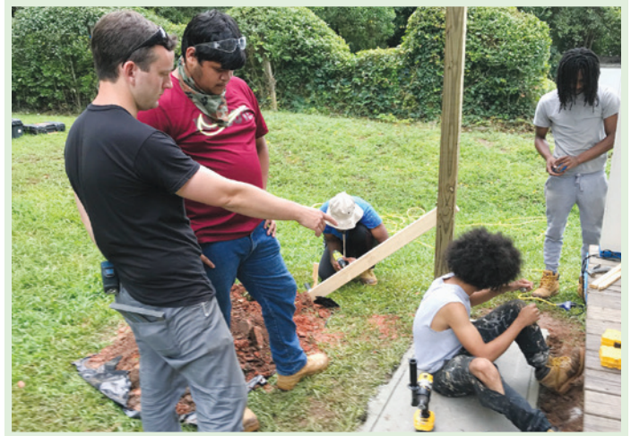
YUB coordinator Lawrence Jones instructs the students on a porch repair project.
